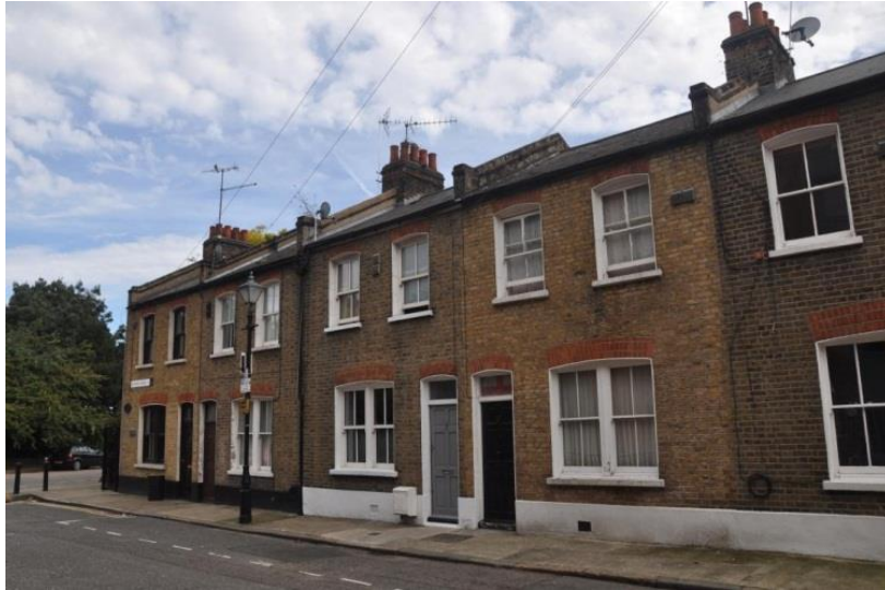
Blondin Street (above): The party walls project through the slope of the roof. Earlier and mid nineteenth century houses were built with roofs of gentle pitch; later nineteenth century houses were built with steeper roofs.
