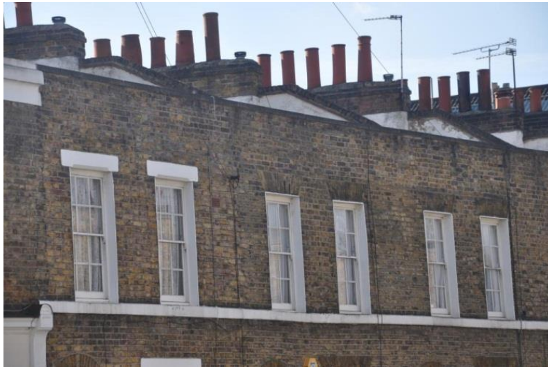
Chasely Street, the modified London roof is visible from the street (above).
