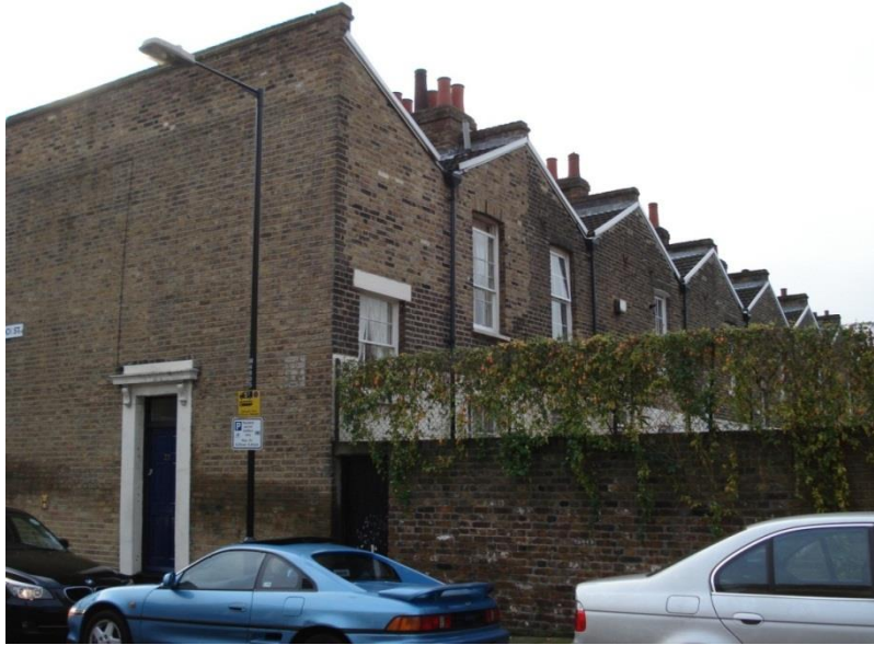
Rear of Aston Street from Matlock Street London (or Butterfly) roof – rear elevation (above): The parapet is omitted from the rear elevation of houses with London roofs exposing the distinctive pattern of gables and valleys to view.
