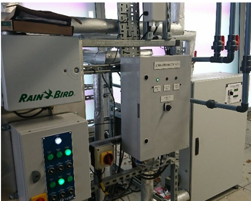
Plate 19: Aqua storm control system, 10 Fenchurch Avenue
