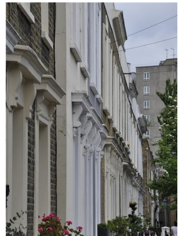
Kenilworth road The replaced consoles in the house to the left have lost the character of the original ornate consoles
