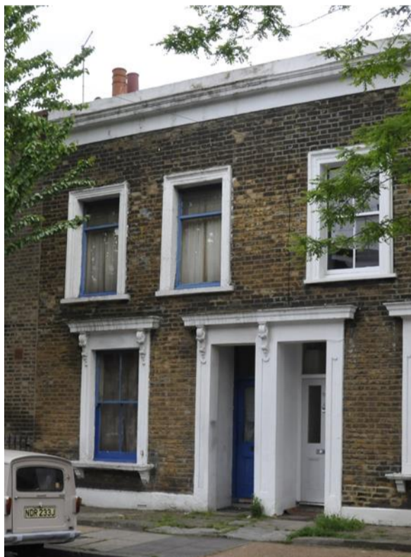
Zealand Road loss of sash windows and stucco console brackets
