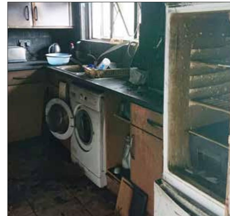
The damage caused by the fire in a Sidney Street property
