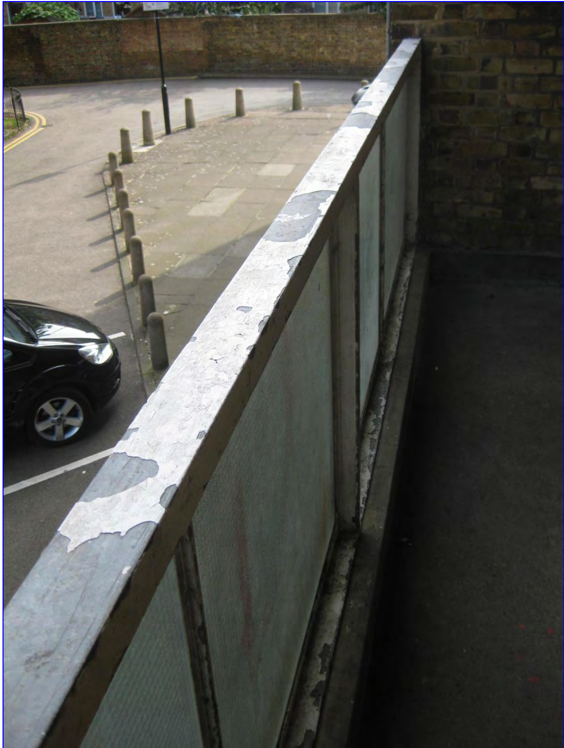
Photograph 18: Example of deteriorated paint coatings to handrail glazing system on walkway.
