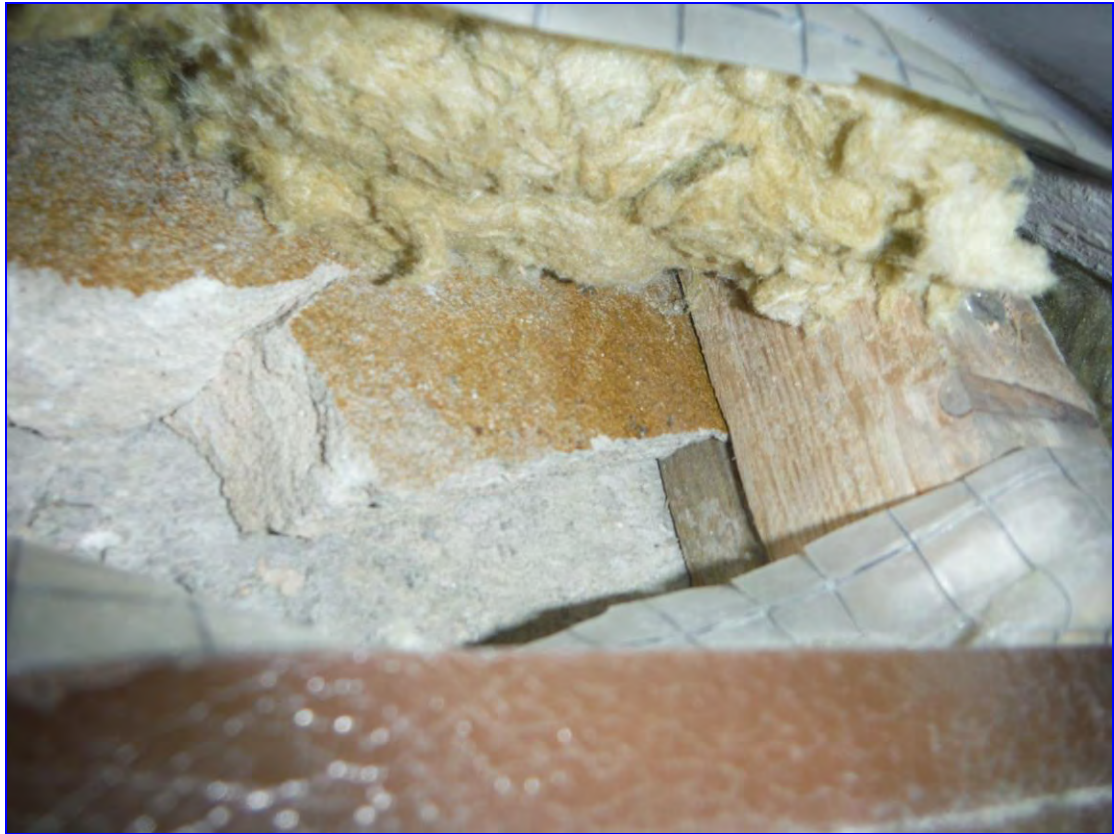
Photograph 27: As previous photograph but opened further revealing timber framework secured back to concrete. Here a render layer behind the insulation is also apparent.
