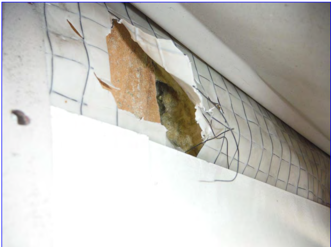
Photograph 23: A closer view, as previous photograph, showing insulation dug out to concrete behind.
