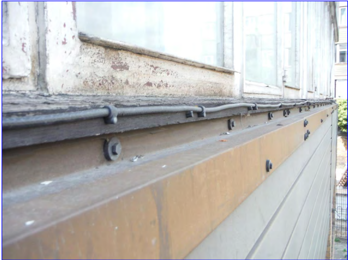
Photograph 25: General view showing typical fixing of cladding at timber work directly below window openings.
