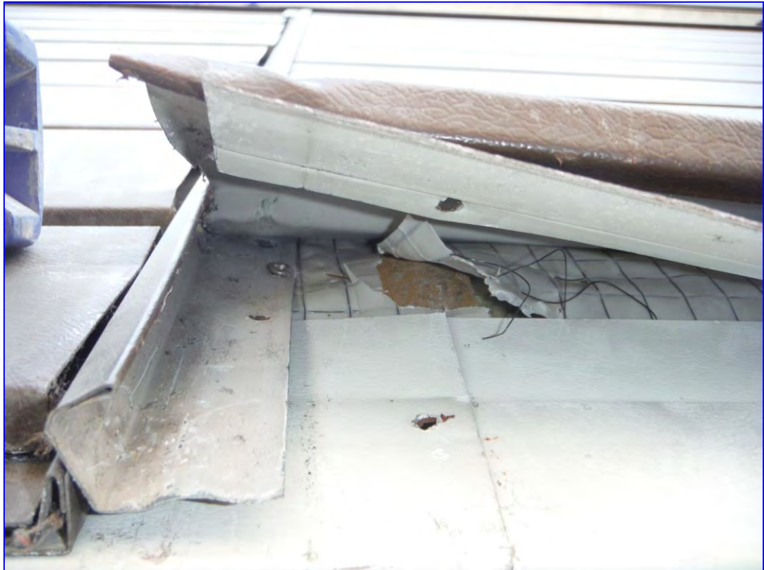
Photograph 22: View showing metal cladding with reinforced sheet behind, over wall insulation (broke through to expose it).
