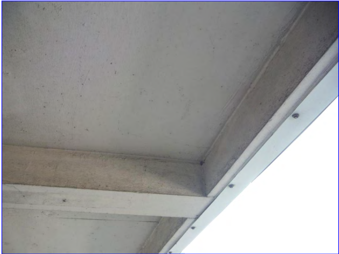
Photograph 20: View showing metal cladding secured along base of concrete slab edge. Note concrete exposed - first floor on Lister.
