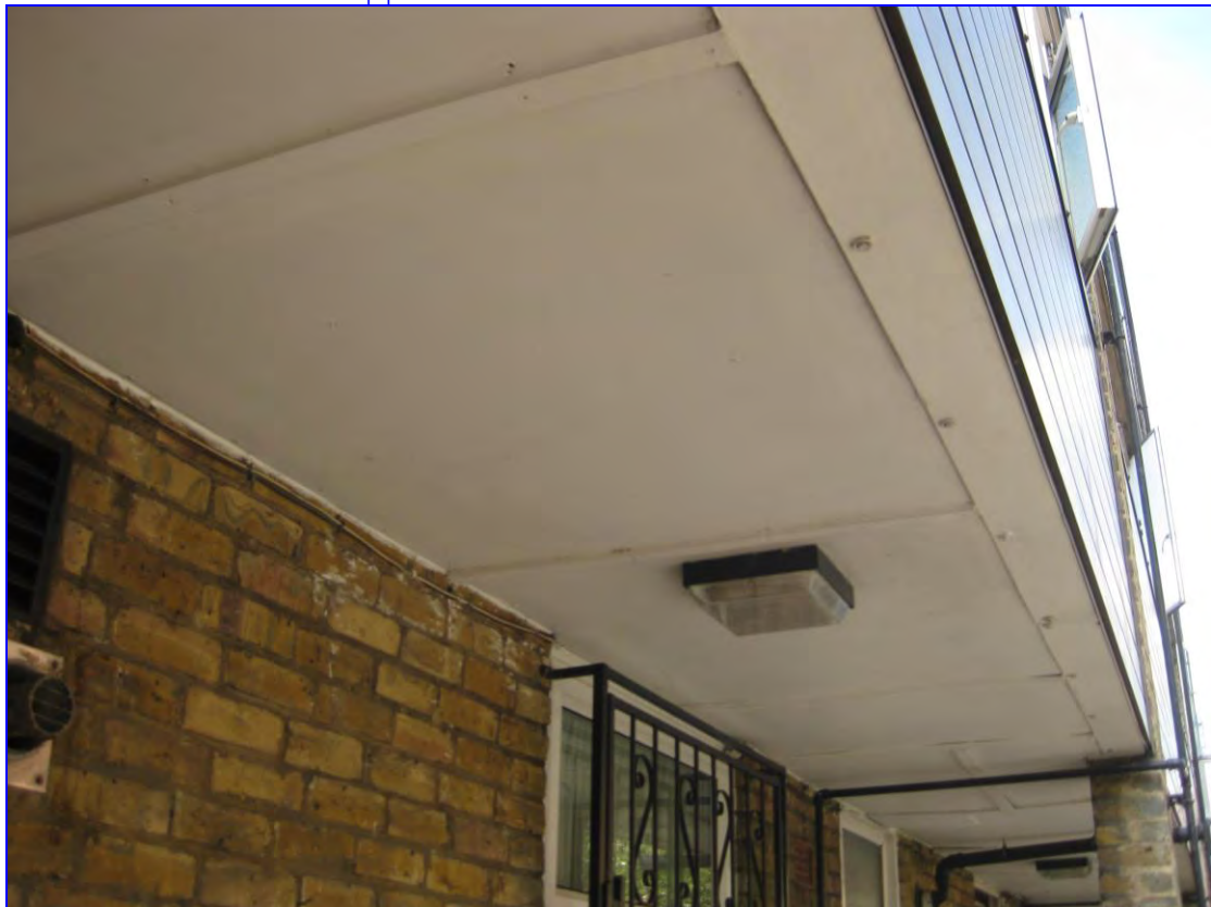
Photograph 28: General view of underside at walkway to Treves, with boarding across the soffit.
