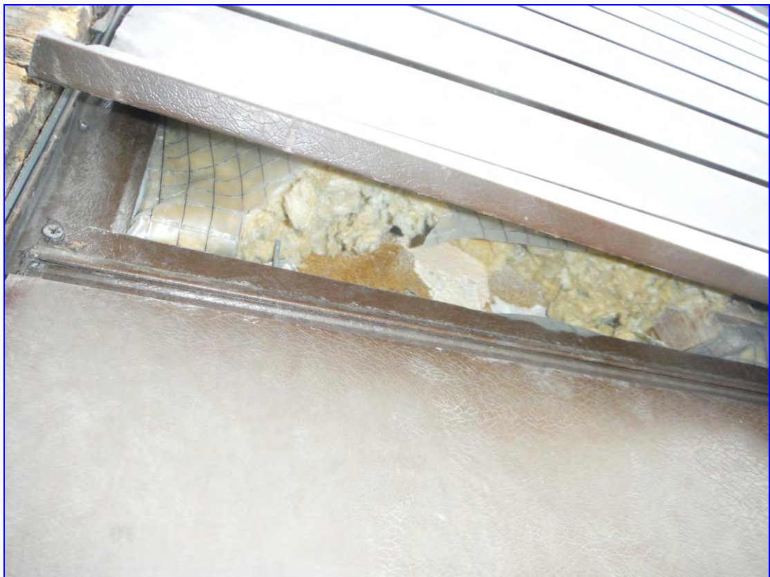
Photograph 26: Another opening up revealing insulation covered by reinforced sheet (on Treves House).
