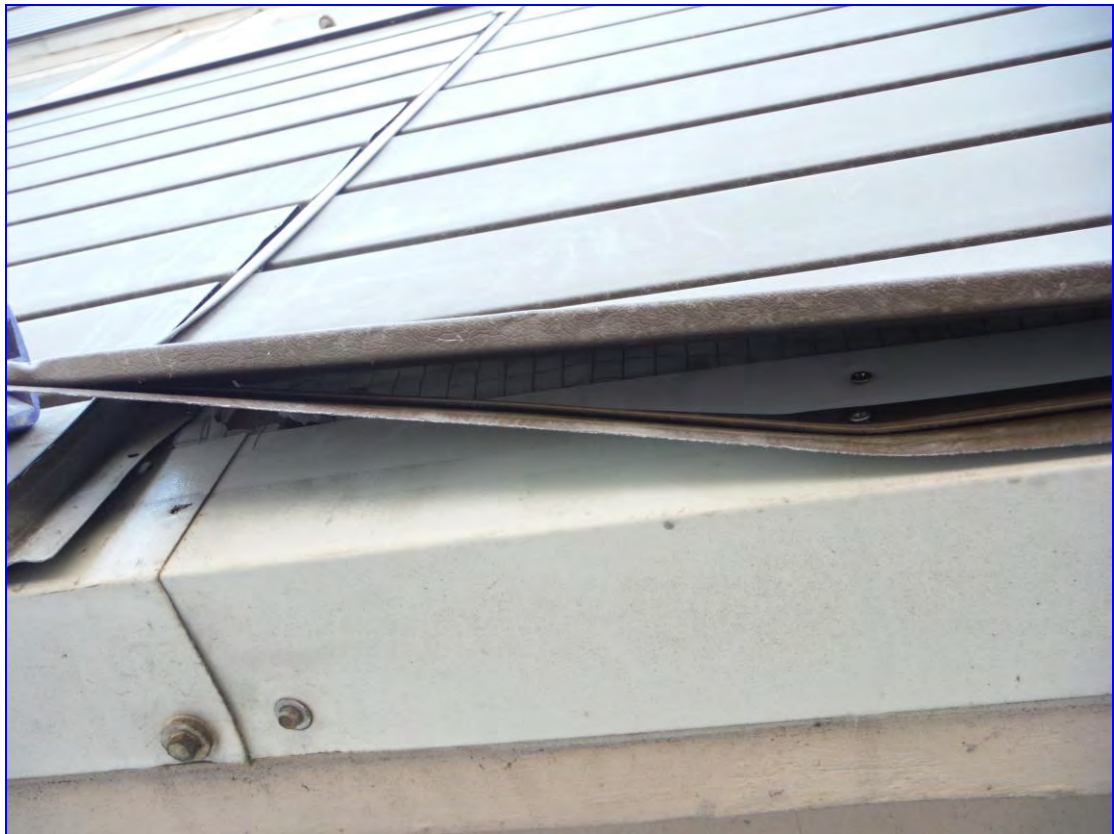
Photograph 21: As lower section of metal cladding lifted revealing edge strip over concrete.
