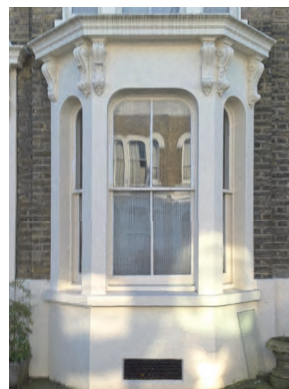
A typical bay window surround (although window horns are missing)
