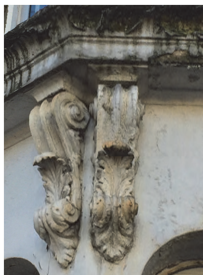
Decorative consoles deteriorate when not well maintained
