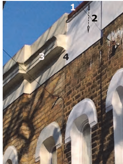
Missing cornice could be renovated using the adjacent cornice as a template
