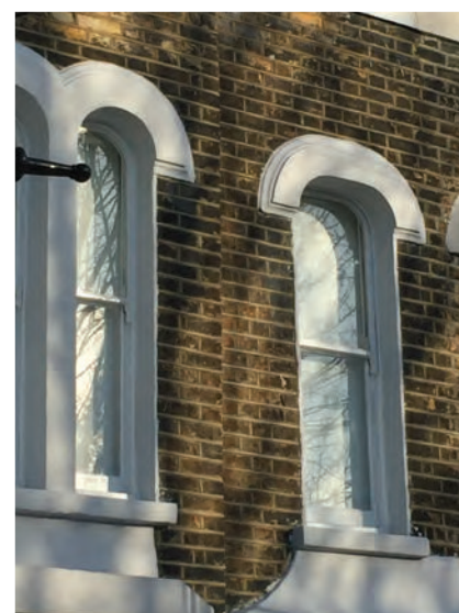
The curved stucco over the bay window was a typical detail but many are lost
